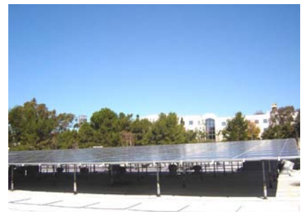
Solar panels on the rooftop of IBEW Local 569, San Diego, California.
