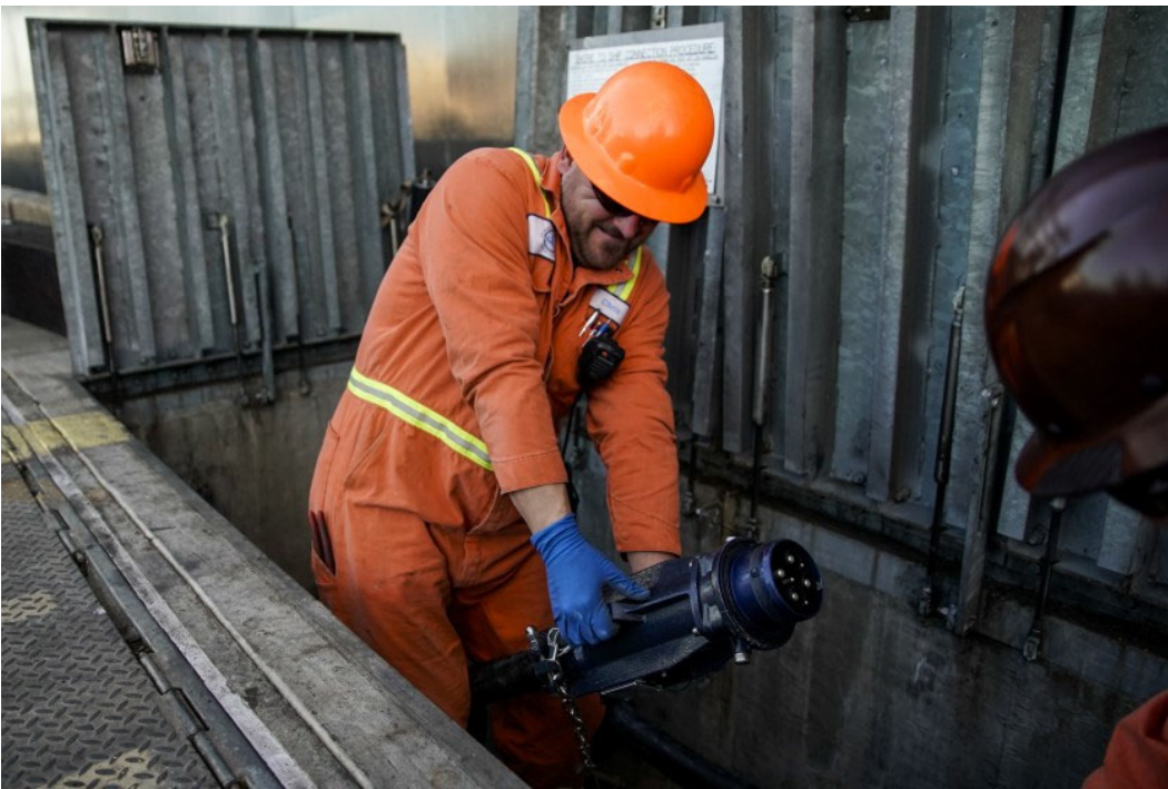
Crane mechanics prepare to connect container ship Yang Ming Movement to the TraPac terminal power grid.
